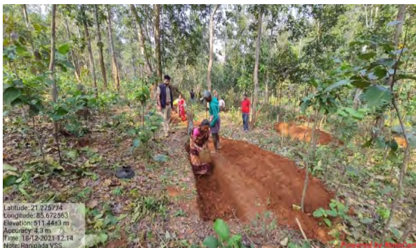
Staggered Trench at Ranipada VSS, Keonjhar WL Division
